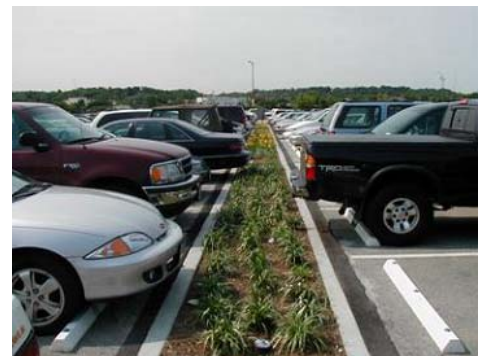
Bioswale or stormwater rain gardens should be considered for larger parking areas.
